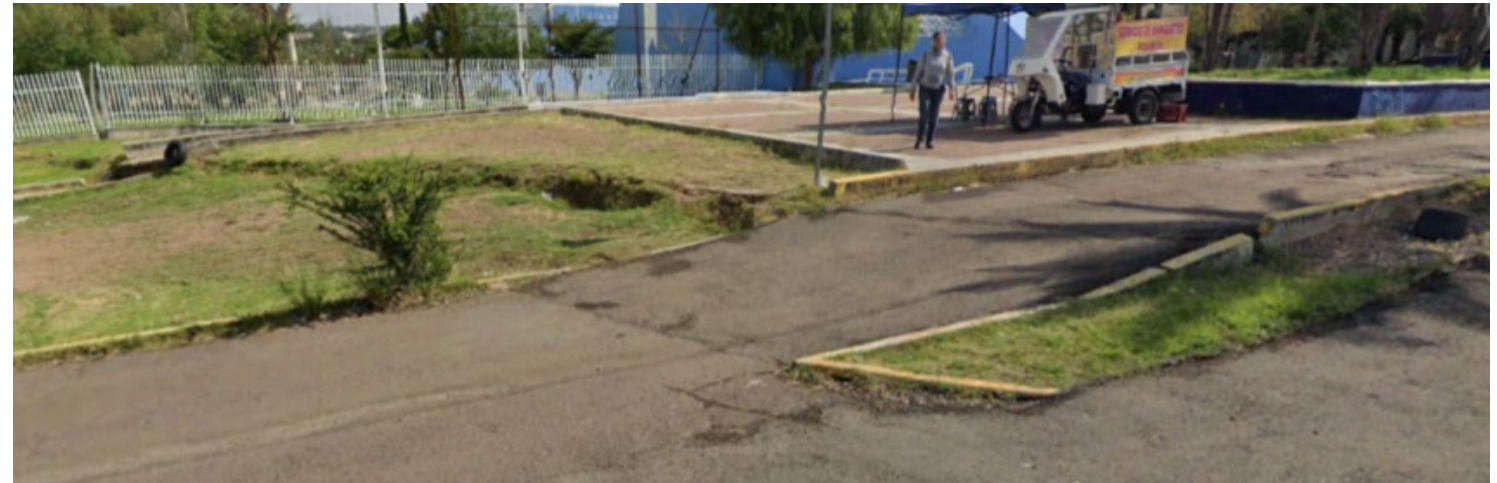
Fissured and ramped urban roads and ground due to surface faulting in Aguascalientes (©INEGI 2020)
